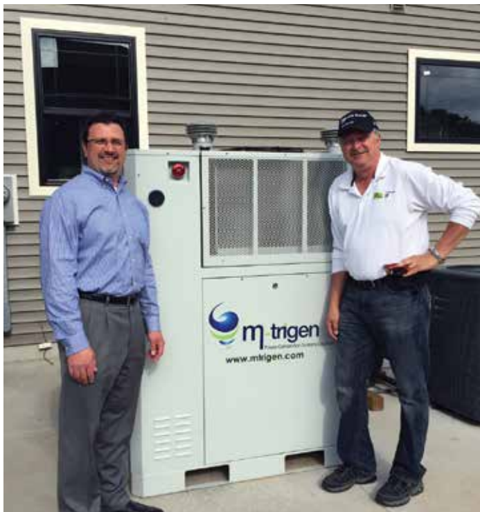
Rob Gryczon, DTE Energy Co., and Robert Fegan, project manager of the micro CHP unit at the Traverse City, Michigan, home at the time it was installed.
